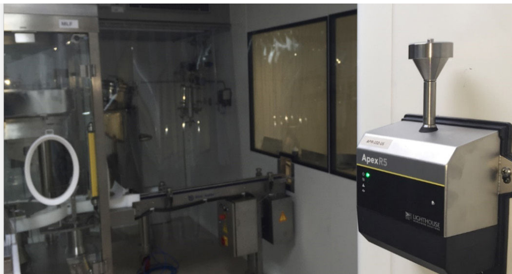
Remote Particle Counter in Grade B/ISO 7 Cleanroom
